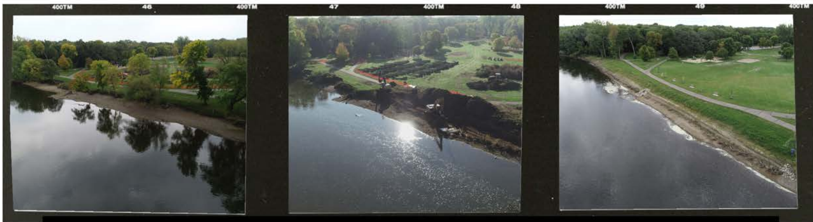
Drone photos before, during, and after construction of a Streambank Project at Otsego County Park.
