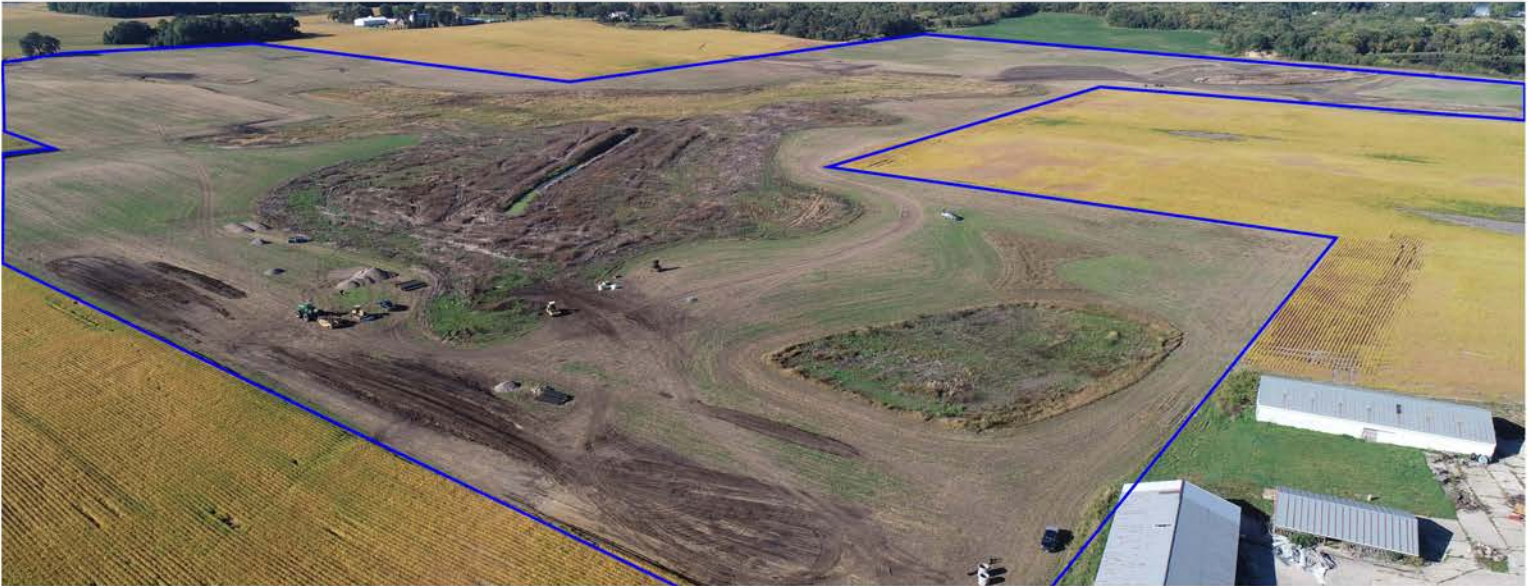
District staff, in partnership with BWSR, and the Wright County Drainage Authority, coordinated with the landowners to abandon a portion of County Ditch 20, enabling the wetland restoration and native prairie for the generation of wetland credits. The easement totals approximately 118 acres (shown in blue). Photo taken during construction in the fall of 2024.
